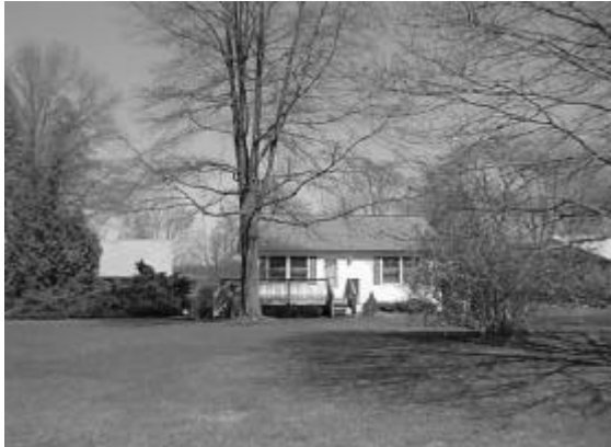
ECHO unit in Three Bridges, Hunterdon County.
